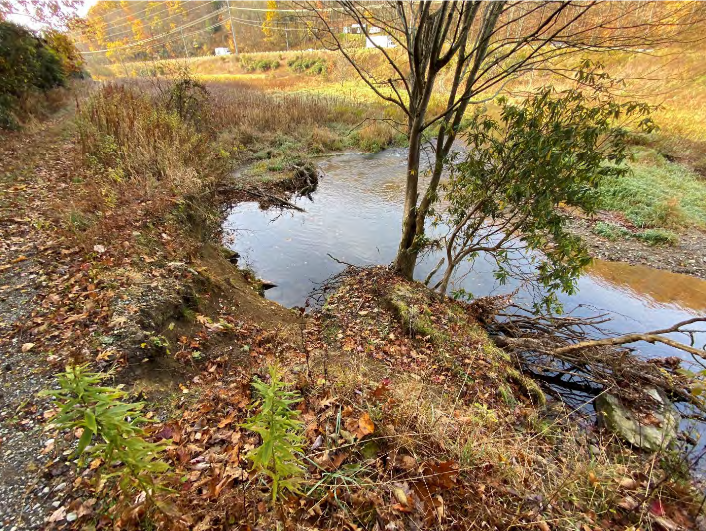
Riverbank Erosion Along Jennifer Ln (Facing South Toward US 321)
